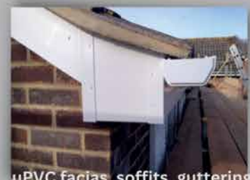
uPVC facias, soffits, guttering
